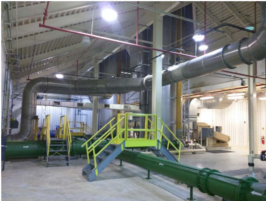
Figure 14-Overview of MRTF interior
