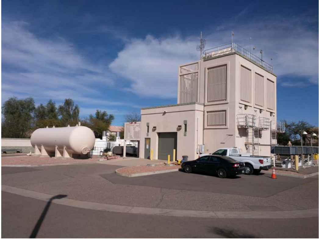
Figure 24- Exterior of Central Groundwater Treatment Facility, looking northeast
