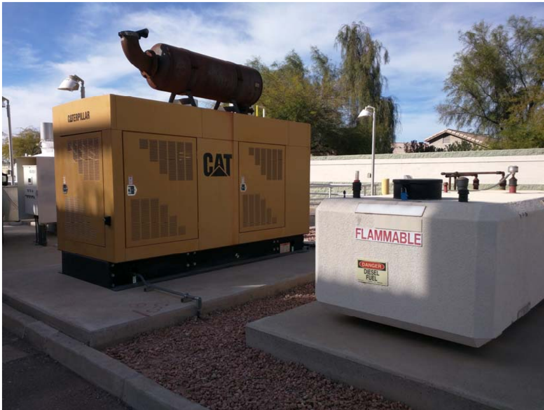
Figure 32-CGTF backup generator and fuel storage
