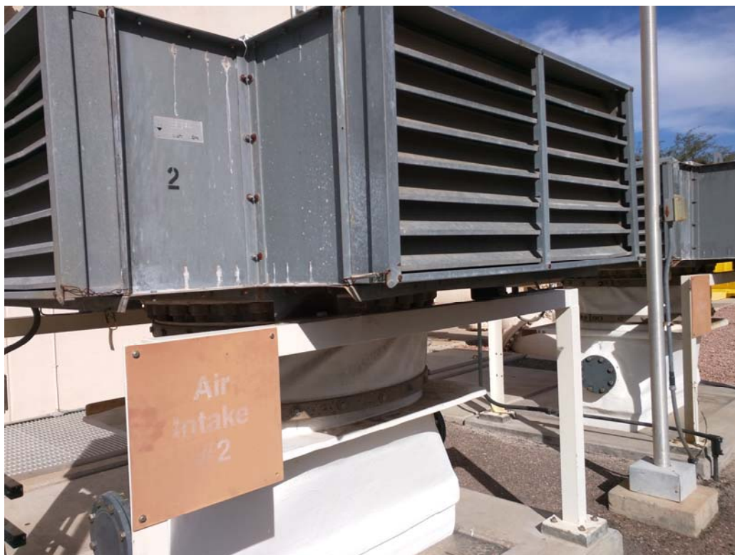
Figure 26- CGTF air intake #2
