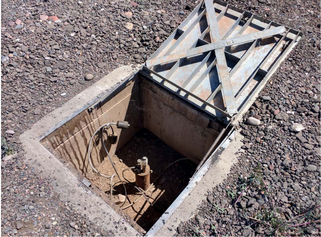
Figure 5- SIBW-11MC well vault
