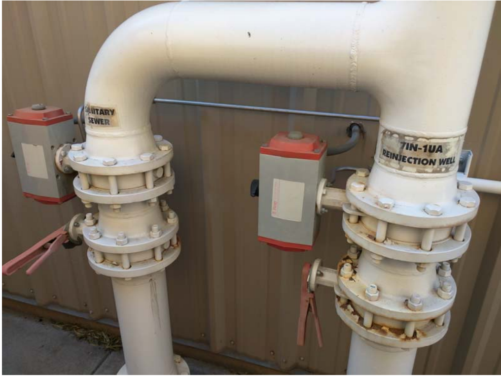
Figure 23-Area 7 reinjection well and sanitary sewer connection
