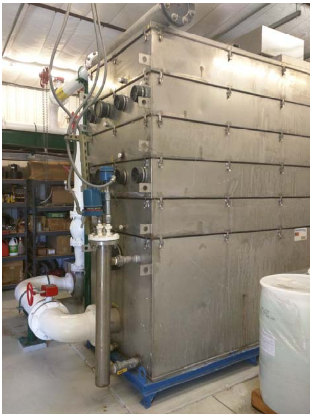
Figure 20-Area 7 air stripper trays
