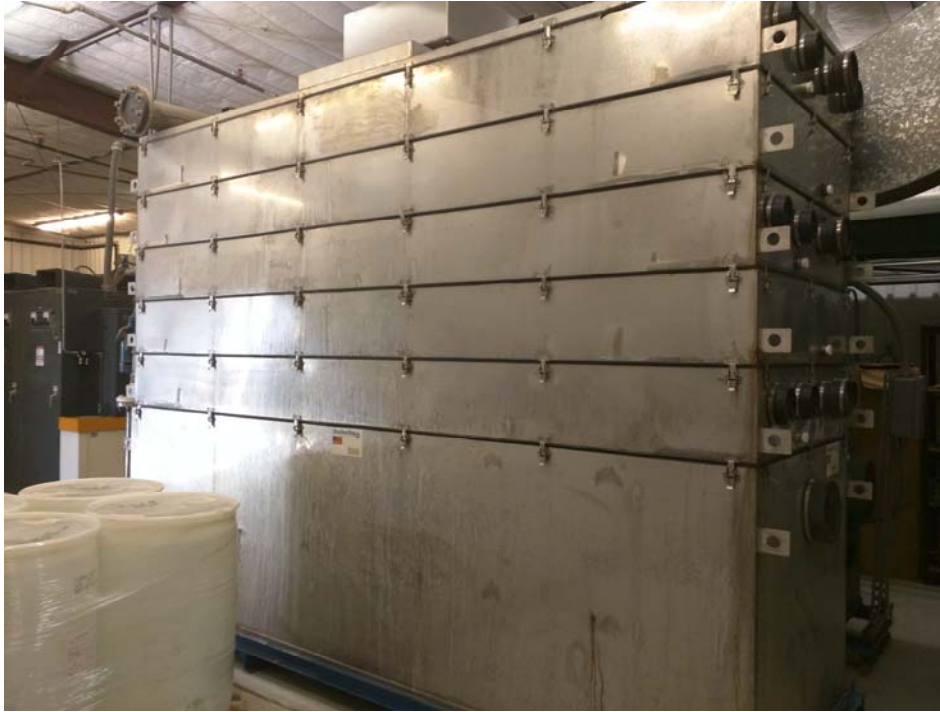
Figure 21-Area 7 air stripper, epoxied weep hole on lower right
