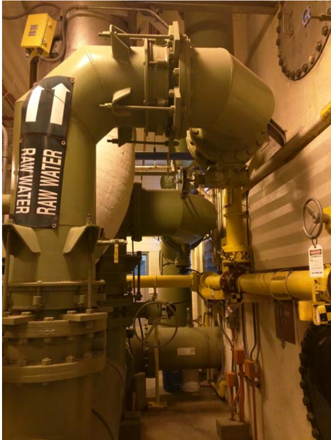
Figure 29-CGTF interior, untreated water intake
