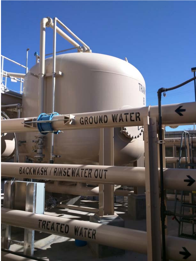
Figure 5-NGTF GAC vessel and piping
