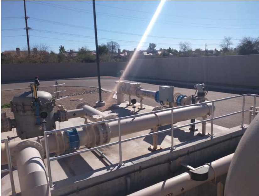
Figure 3-NGTF groundwater intake piping
