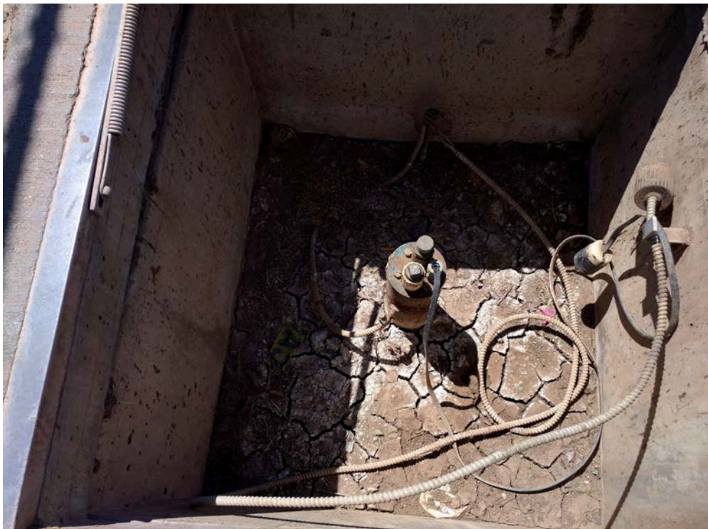
Figure 8- SIBW-13MC well vault interior
