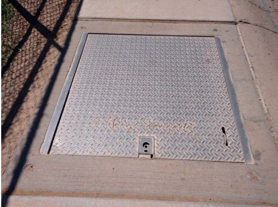
Figure 9-SIBW-13MC well vault exterior
