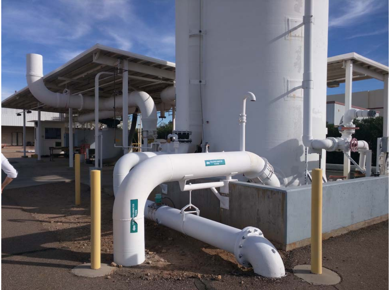
Figure 33-Area 12 air stripper tower, looking southeast
