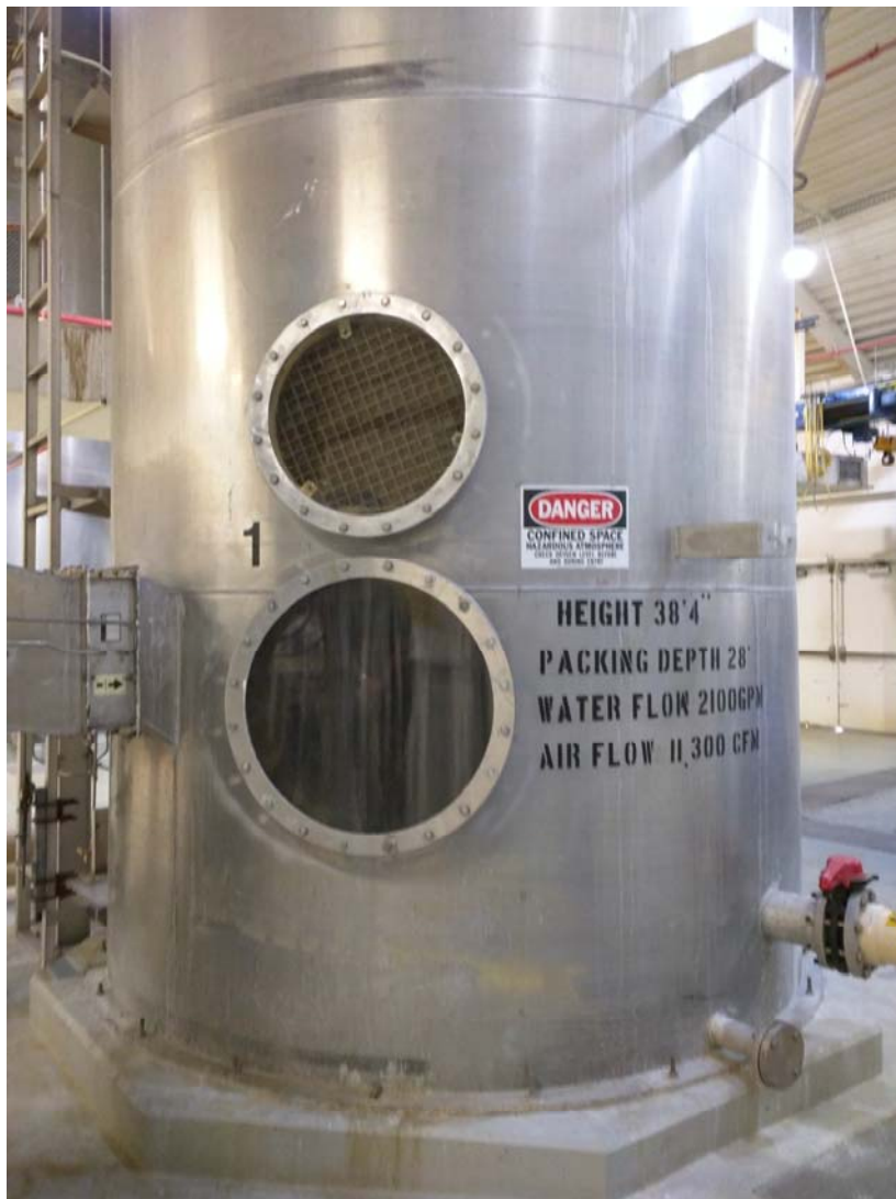
Figure 10-MRTF air stripper tower
