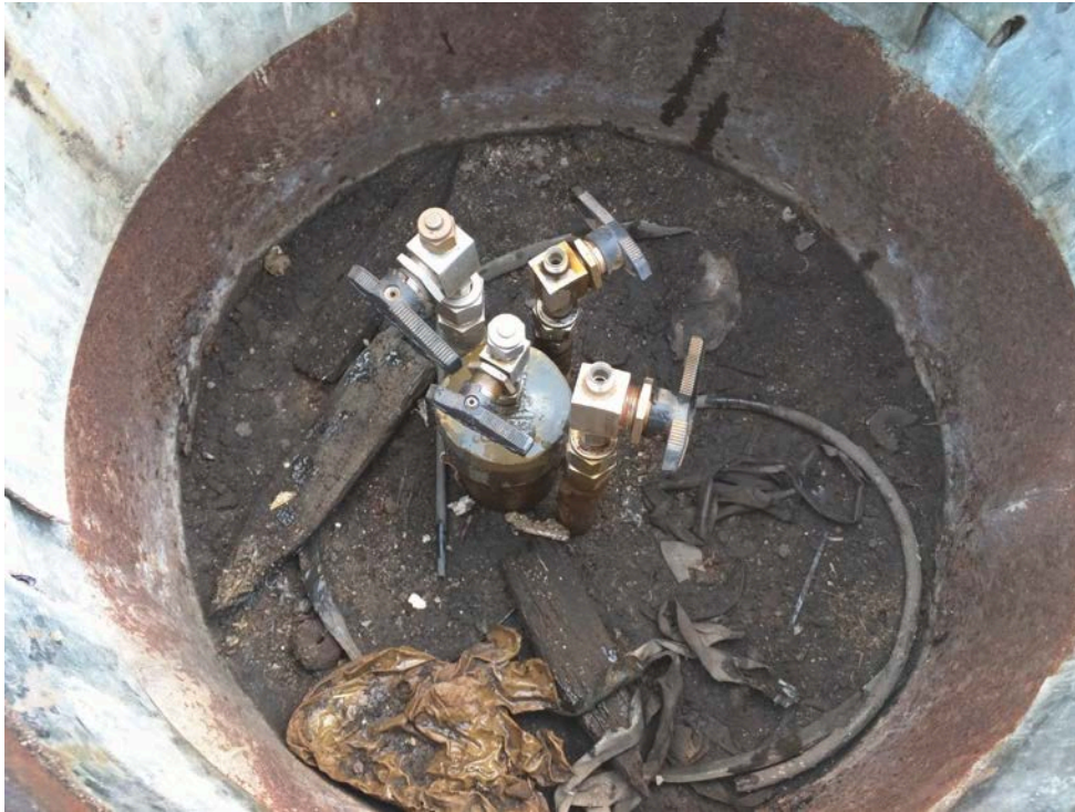
Figure 1- SVE system sampling port
