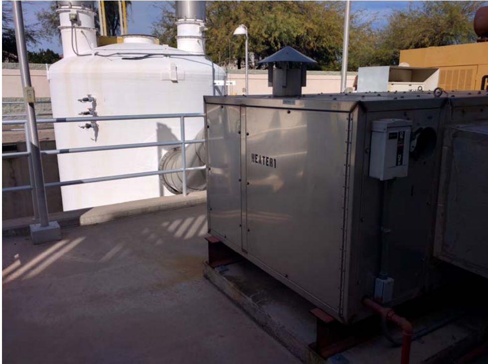
Figure 31-CGTF pre-heater and carbon adsorption vessel
