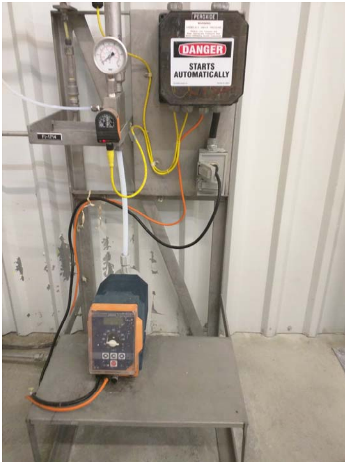
Figure 22-Area 7 metered pump for peroxide
