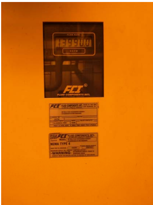
Figure 30- CGTF column #3 flow meter
