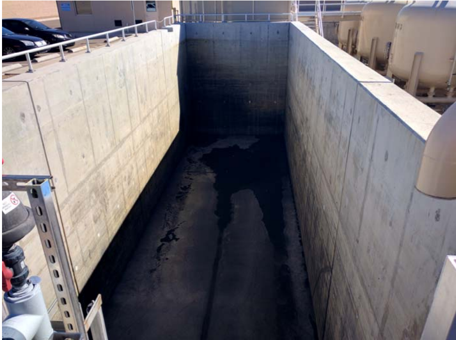
Figure 7-NGTF Backwash holding tank
