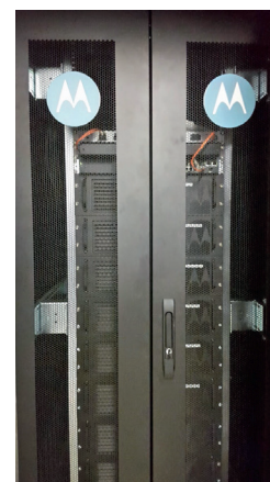
MOTOTRBO DR 3000 repeaters in indoor rack closet
